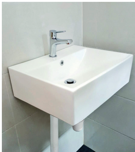
Wash basin with tap mixer
