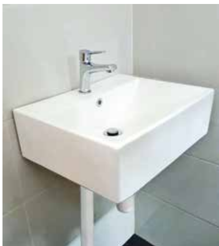
Wash basin with tap mixer
