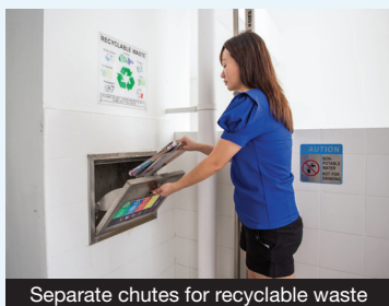
Separate chutes for recyclable waste
