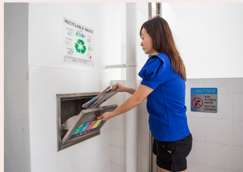
Separate chutes for recyclable waste
